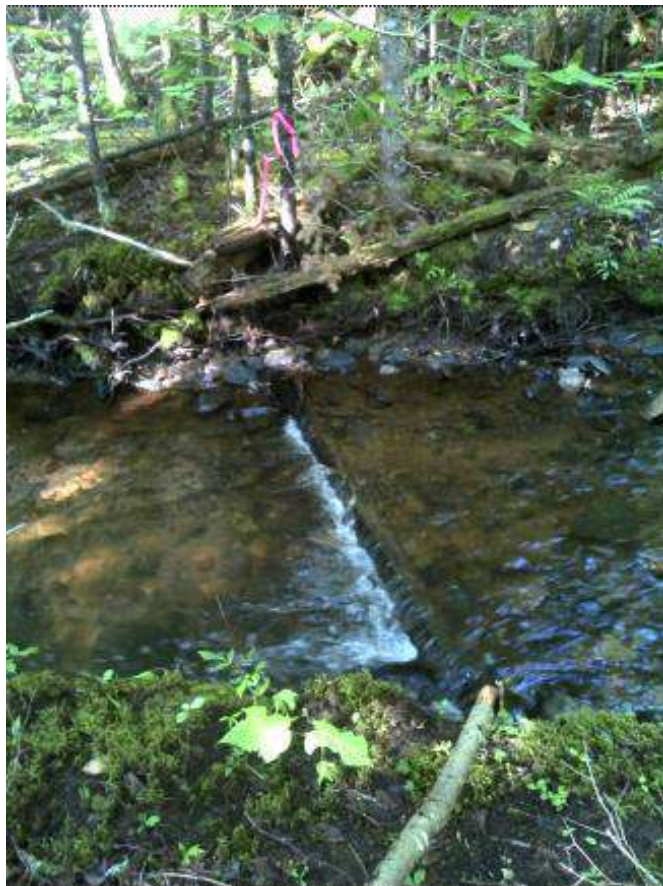
Figure 68. Structure #20 - Before and after picture of the maintenance completed on a diggerlog.
