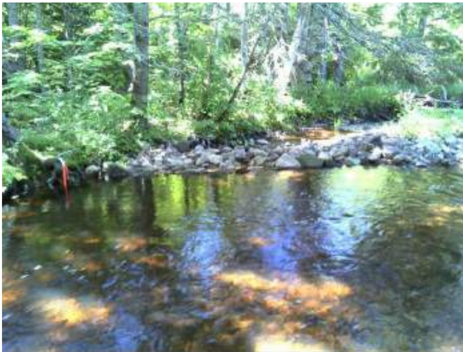
Figure 225. Structure #39 Channel Blocker constructed with rocks - before and after pictures of completed maintenance.
