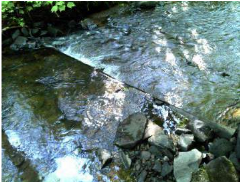
Figure 59. Structure #11 - Before and after picture of the maintenance completed on a digger log.
