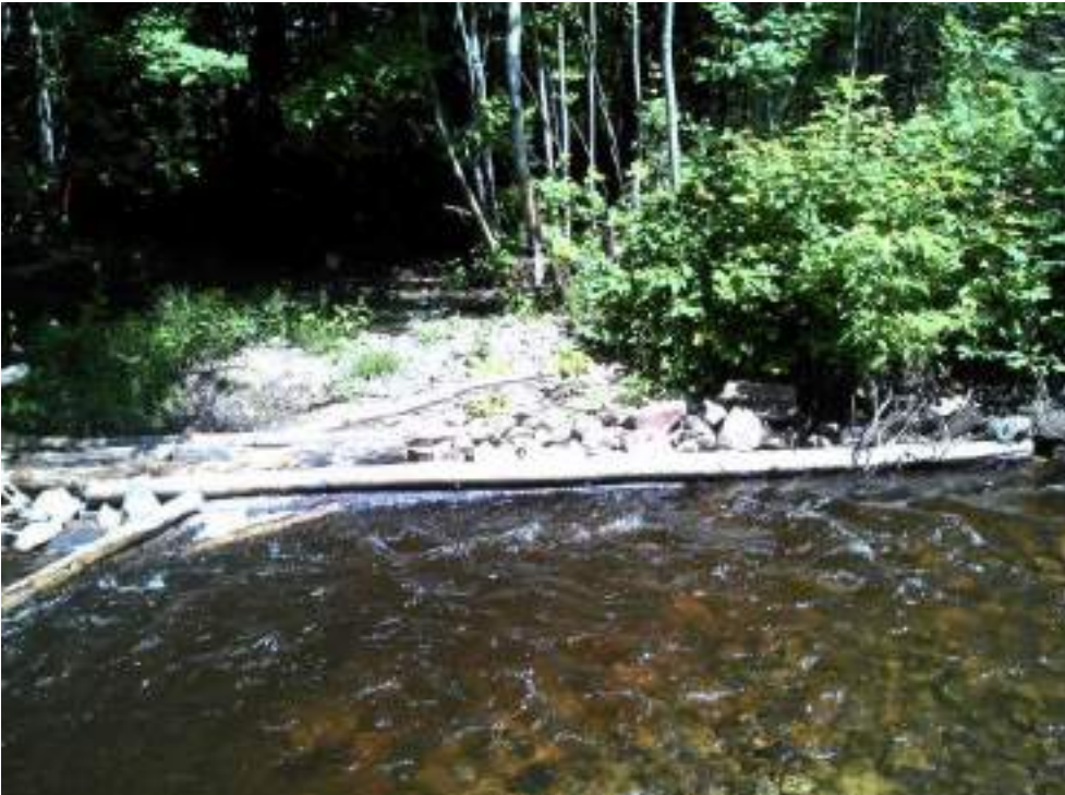
Figure 227. Structure #41 Two Tier Channel Blocker - before and after picture of completed maintenance.
