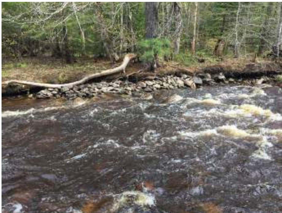
Figure 244. Structure #58 Deflector - requires a rebuild.
