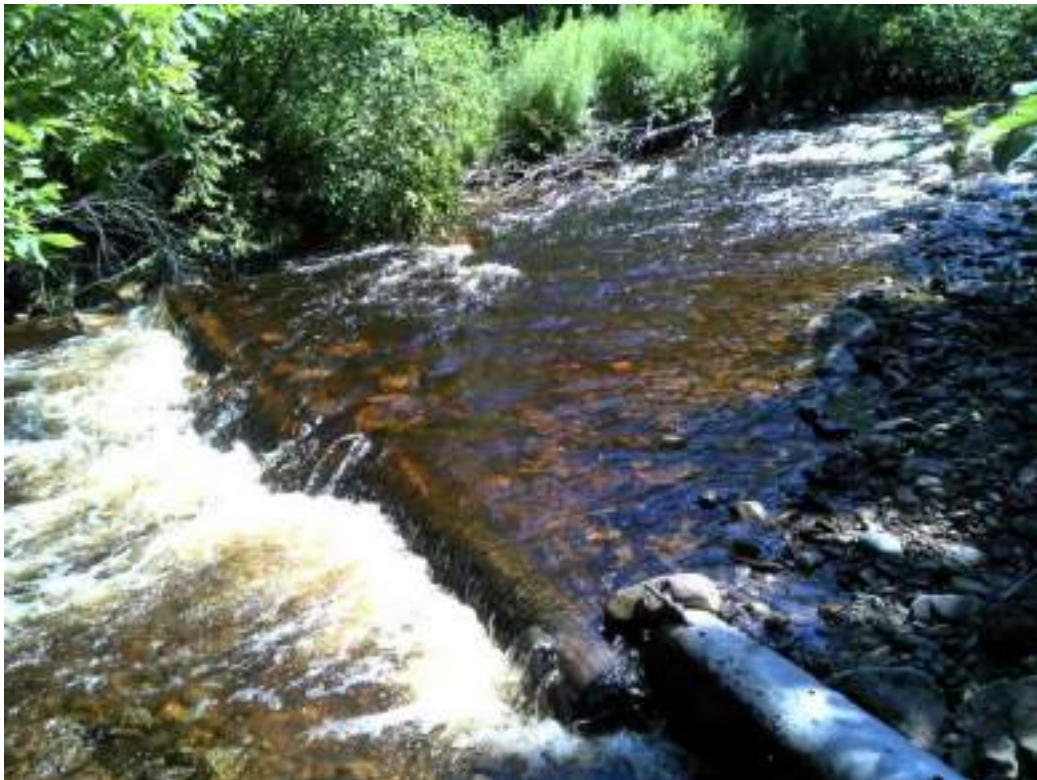
Figure 210. Structure #24 Diggerlog - before and after picture of completed maintenance. This log was cut in half during installation due to its weight.
