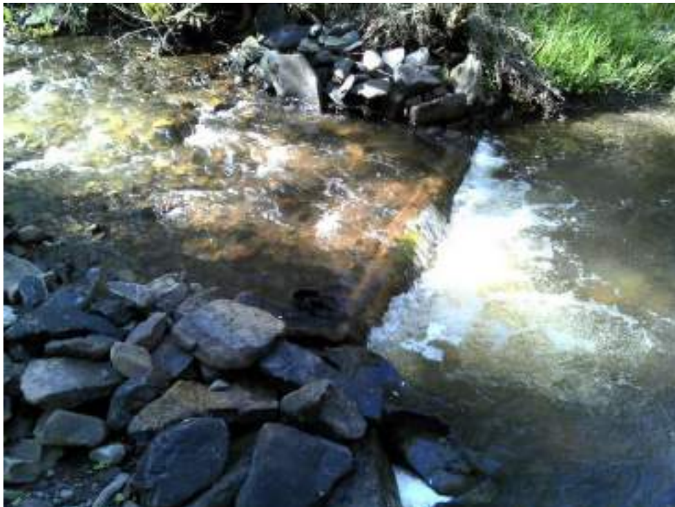
Figure 18. Showing the before and after photos of a digger log - structure #8 downstream from the road.
