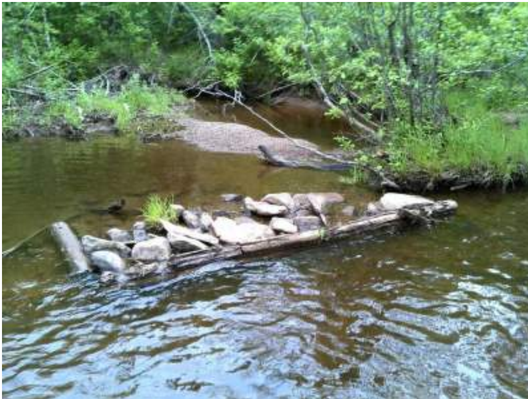
Figure 154. Deflector #7 - no maintenance performed. The channel started flowing around the structure, flooding it with water.
