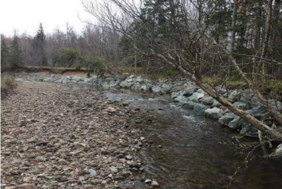
Figure 192. Structure #7 Armour Stone - bank stabilization
