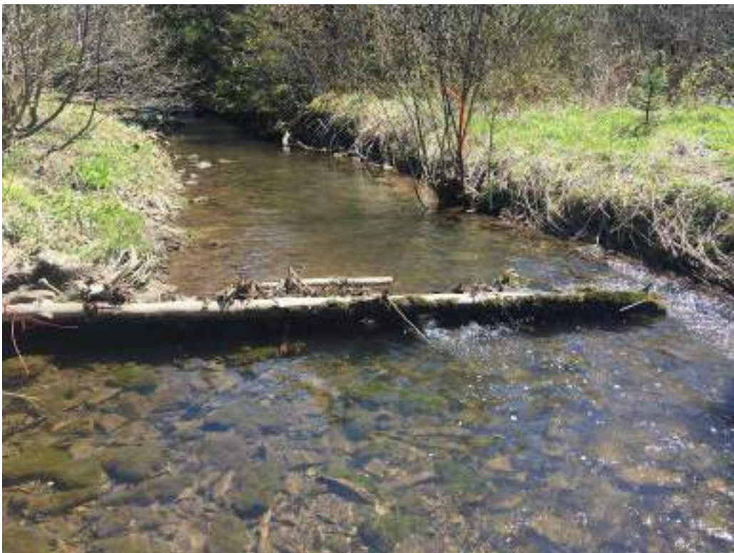
Figure 83. Structure #8 - diggerlog that needs a replacement. This is the last structure on the downstream side of Smithville Road.
