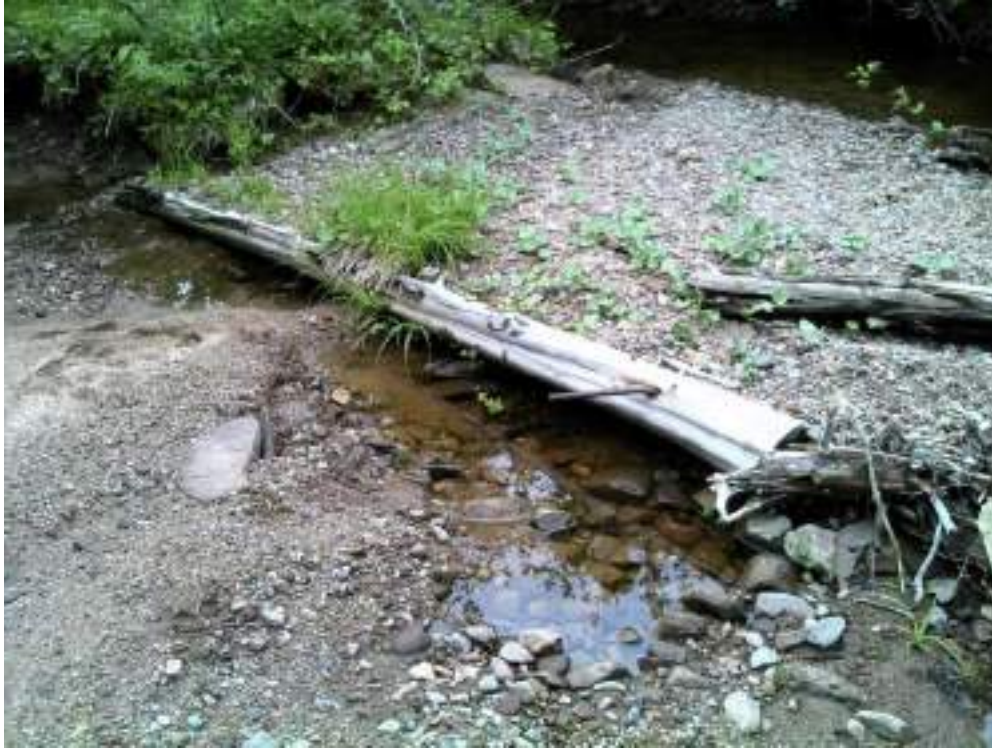
Figure 166 - Diggerlog #5 - the channel had changed course and the structure is no longer in the channel. This structure needs to be replaced, and repositioned.
