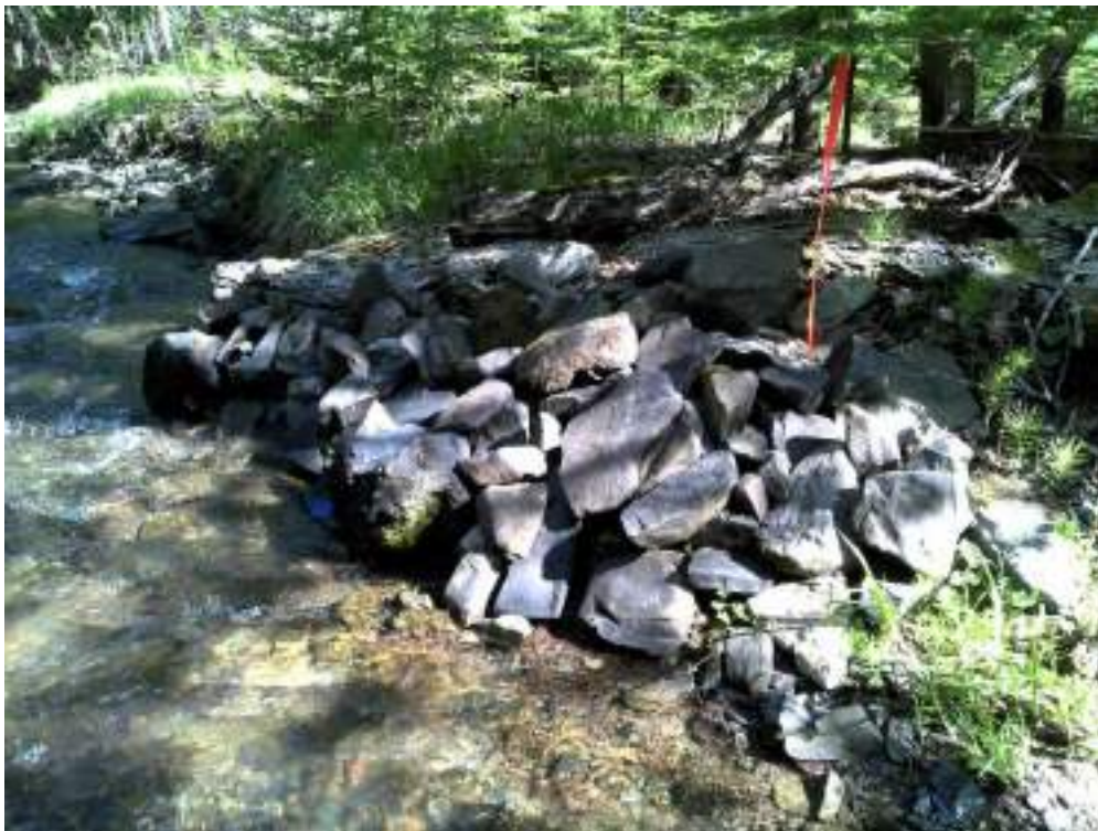
Figure 22. Showing the before and after pictures of a bank stabilization structure #12 - downstream from the road.
