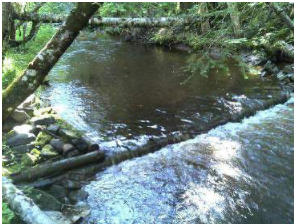
Figure 176. Structure #5 - After picture of the maintenance completed on a diggerlog and deflector structure.
