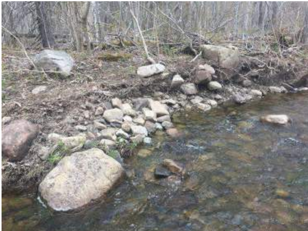
Figure 235. Structure #49 Deflector - requires full rebuild.
