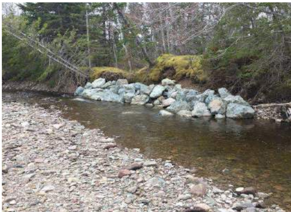
Figure 199. Structure #13 Armour Stone - bank stabilization.
