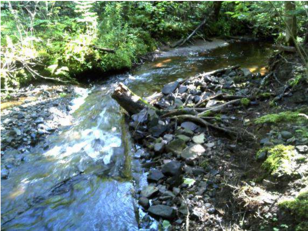
Figure 54. Structure #6 - before and after picture of the maintenance completed on a deflector.
