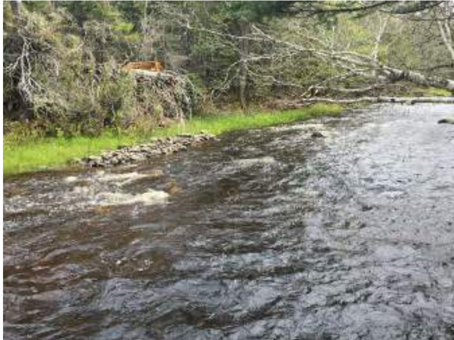
Figure 243. Structure #57 Deflector - upstream from the bottom of Campbells road. This structure needs to be rebuilt.
