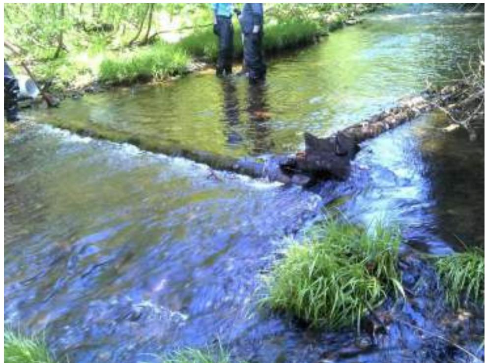
Figure 144. Diggerlog #7 - before and after picture of maintenance performed. This structure is too short and may require a full replacement or permanent extension. Debris materials were added to direct waterflow over the log.
