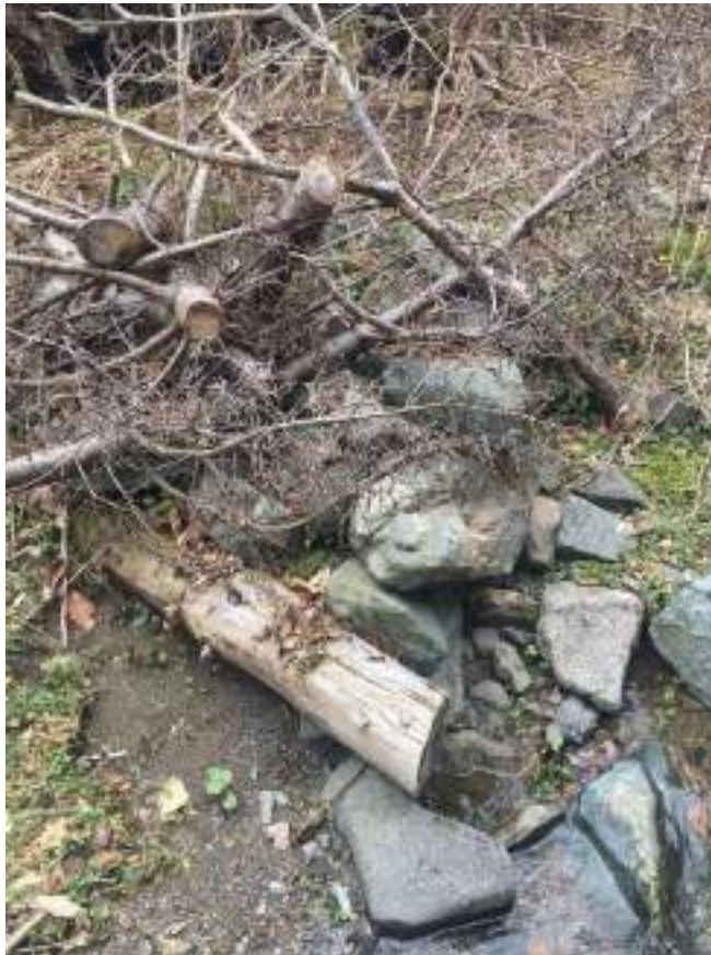
Figure 40. Deflector #13 - structure is no longer in-stream.
