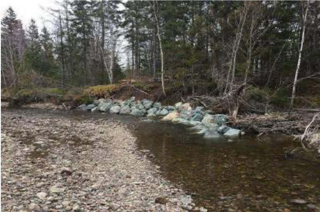
Figure 198. Structure #12 Armour Stone - bank stabilization.
