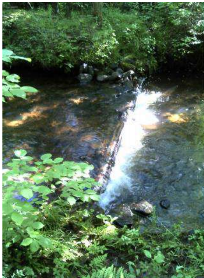
Figure 61. Structure #13 - Before and after picture of the maintenance completed on a digger log.
