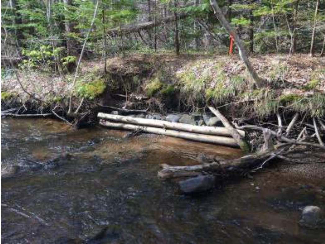
Figure 60. Structure #12 - After picture of the maintenance completed on a two-tier bank stabilization structure.
