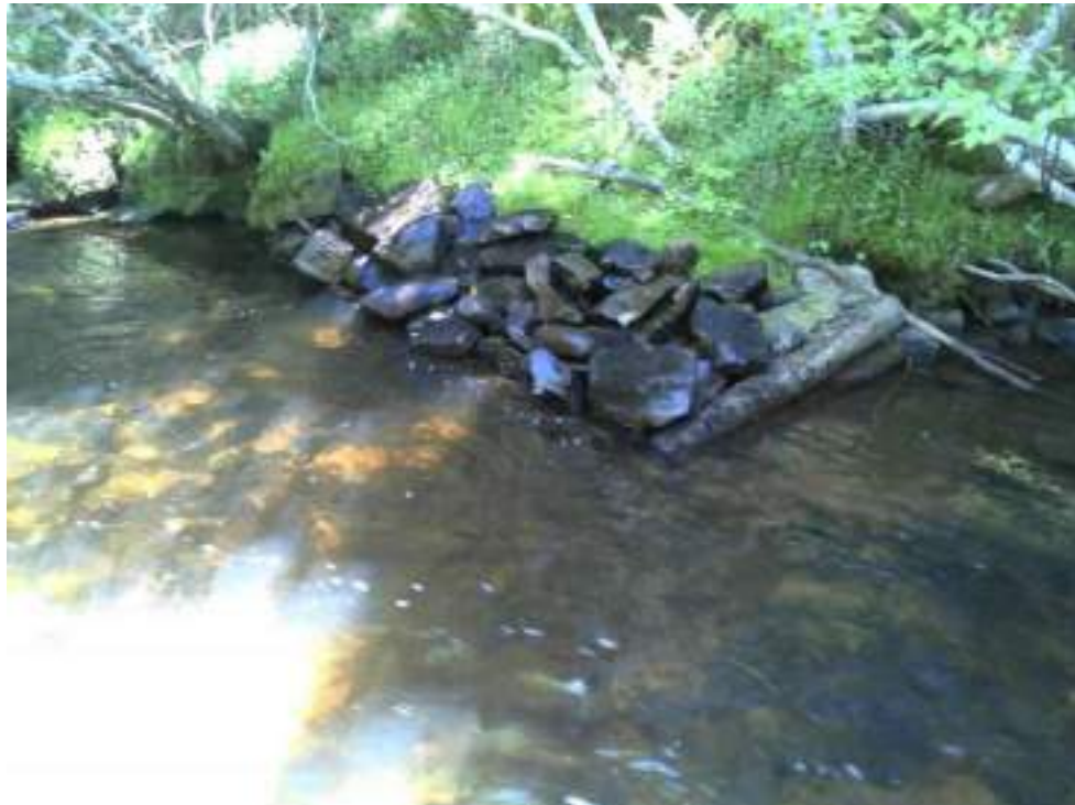
Figure 138. Before and after pictures of the maintenance performed on the furthest upstream structure - Deflector #1.
