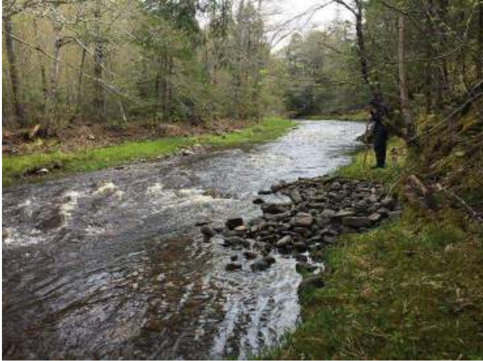
Figure 245. Structure #59 Double Deflectors - requires a rebuild.
