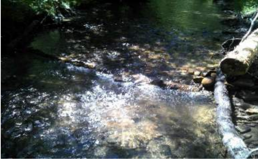
Figure 99. Diggerlog #5 - maintenance was attempted but not successful. This structure may need replacement.
