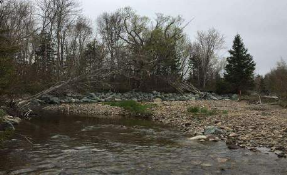
Figure 194. Structure #9 - Armour Stone - bank stabilization
