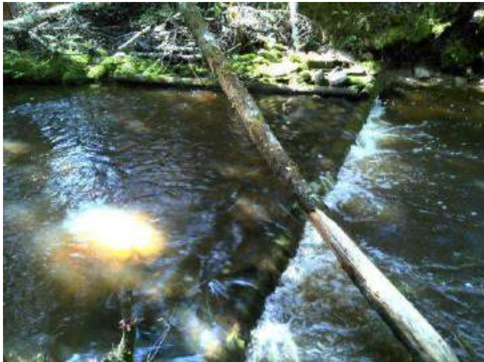
Figure 175. Structure #4 - After picture of the maintenance completed on a digger log and deflector structure.
