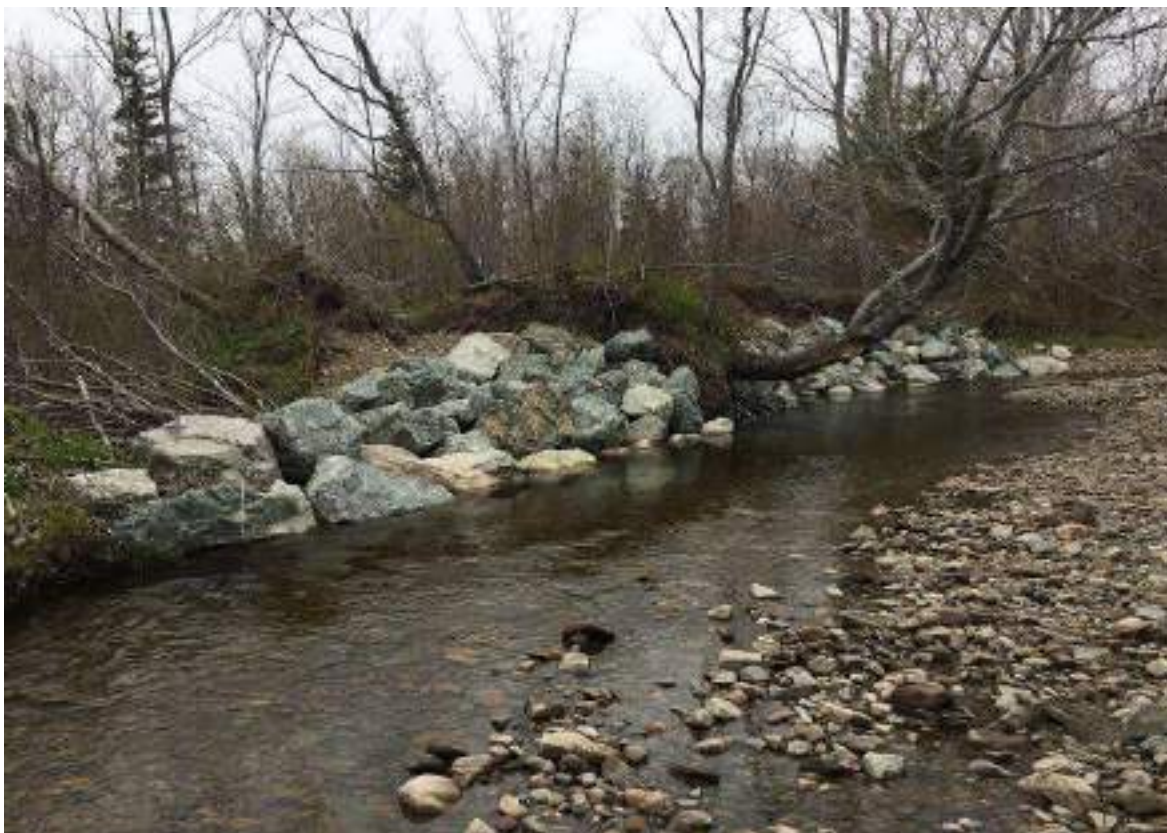
Figure 197. Structure #11 Armour Stone - bank stabilization.
