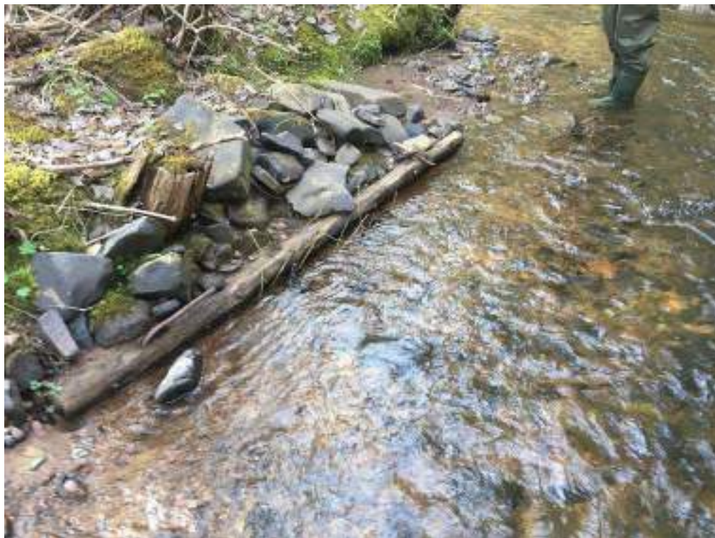
Figure 57. Structure #9 - Before and after picture of the maintenance completed on a deflector.
