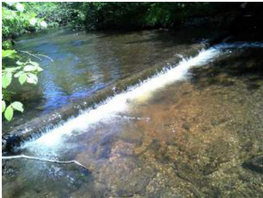
Figure 143. Diggerlog #6 - after picture of maintenance performed. This structure was in very good condition.
