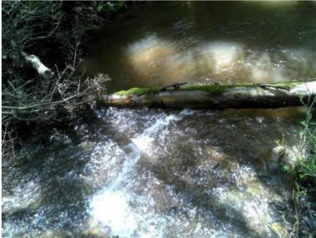
Figure 117. Diggerlog #23 - structure is washed out underneath. No maintenance performed - recommended removal.
