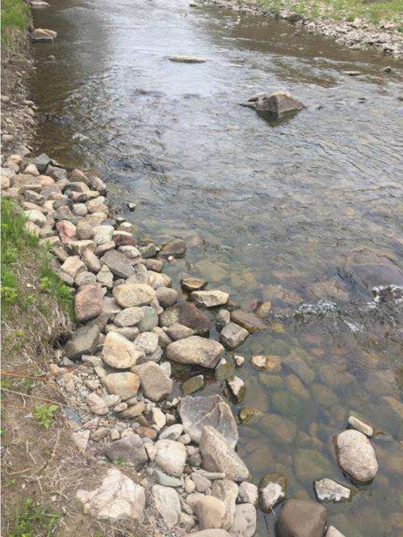
Figure 231. Structure #45 Deflector - requires full rebuild.
