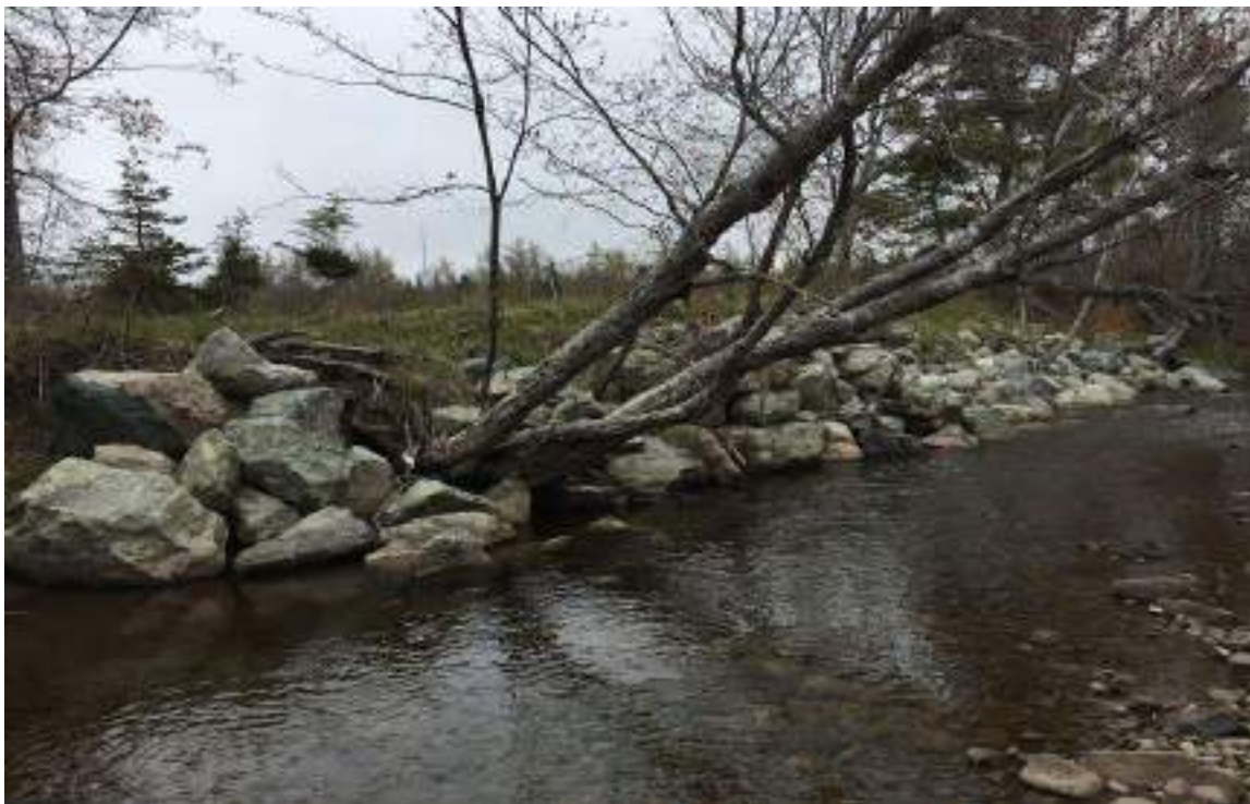
Figure 202. Structure #16 Armour Stone - bank stabilization.
