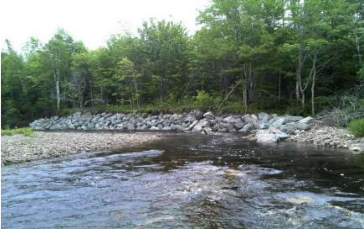
Figure 196. Structure #10 Armour Stone - bank stabilization.
