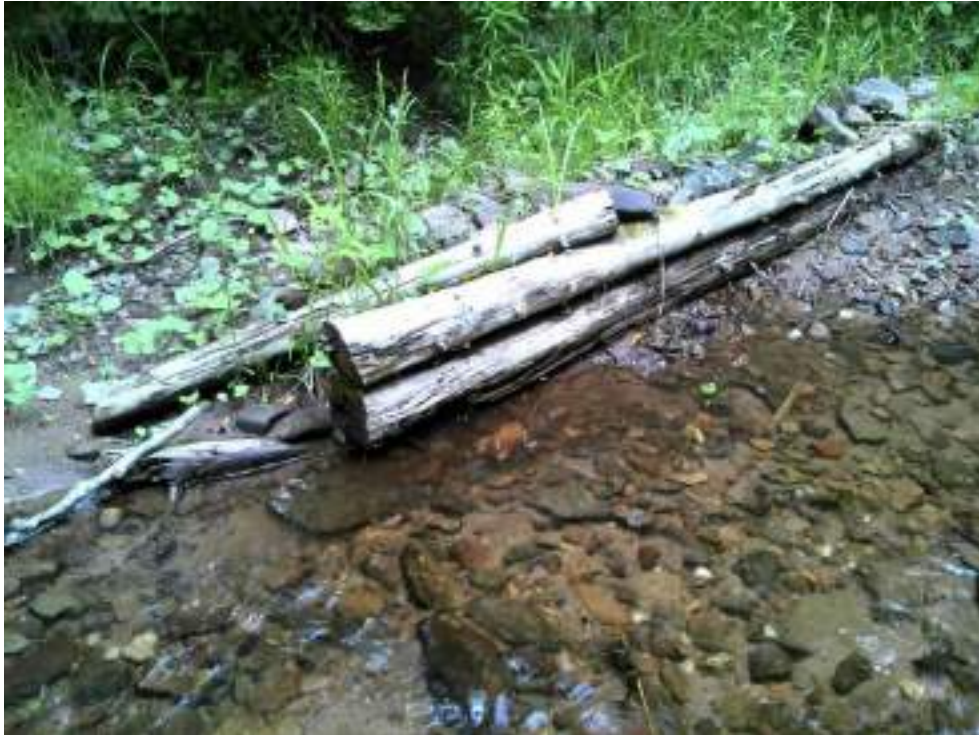
Figure 162. Deflector #1 - this structure is no longer in the channel and needs to be replaced, and repositioned.
