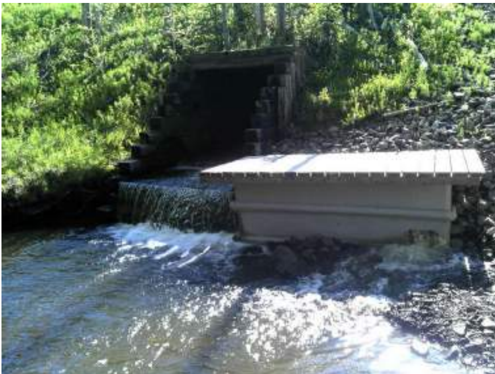
Figure 16. Showing the before and after photos of the fish ladder downstream from the road. The structure was fully blocked up with rock and other woody debris. The fish ladder is now flowing water and is providing upstream access to migrating fish species.
