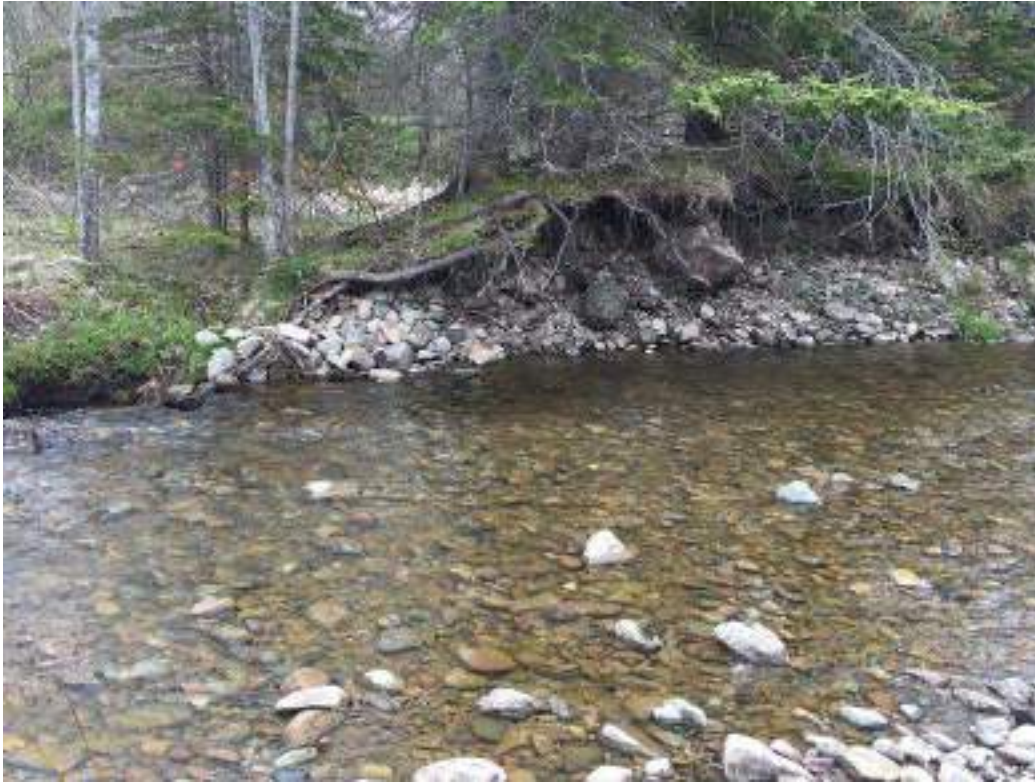
Figure 186. Structure #1 Bank Rock - before picture of maintenance, first structure starting upstream from Route 19 bridge. No after picture taken.
