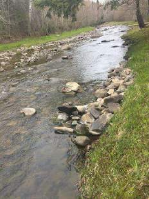
Figure 240. Structure #54 Deflector - requires a full rebuild.
