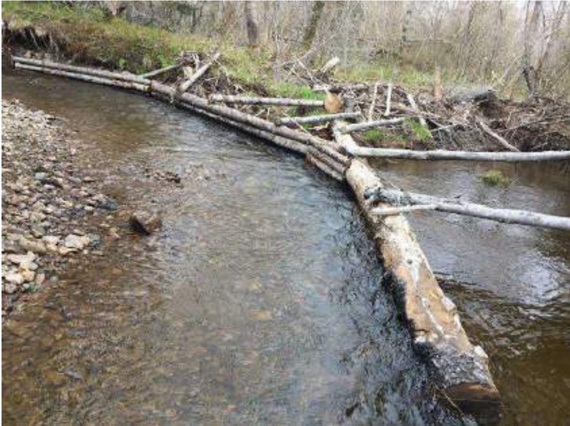
Figure 212. Structure #26 Channel Blocker - no maintenance required.
