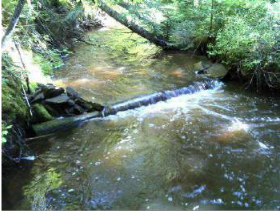
Figure 172. Structure #1 furthest downstream - After picture of the maintenance completed on a digger log.
