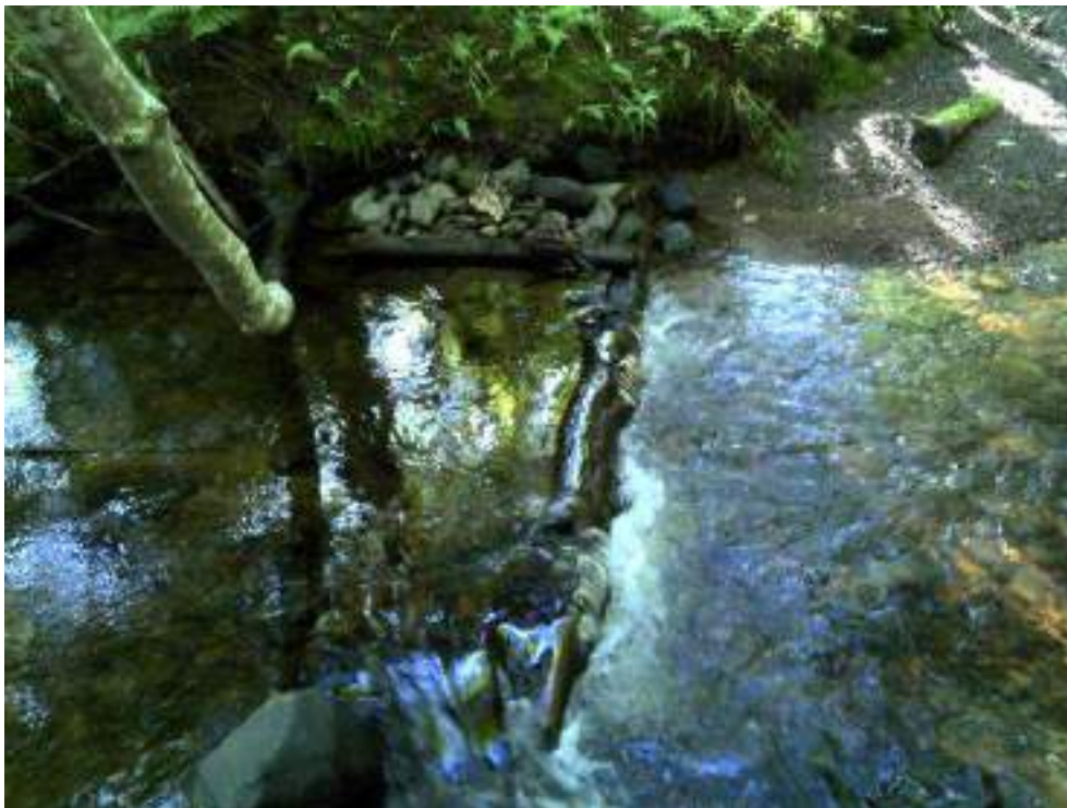
Figure 55. Structure #7 - Before and after picture of the maintenance completed on a digger log and deflector structure.
