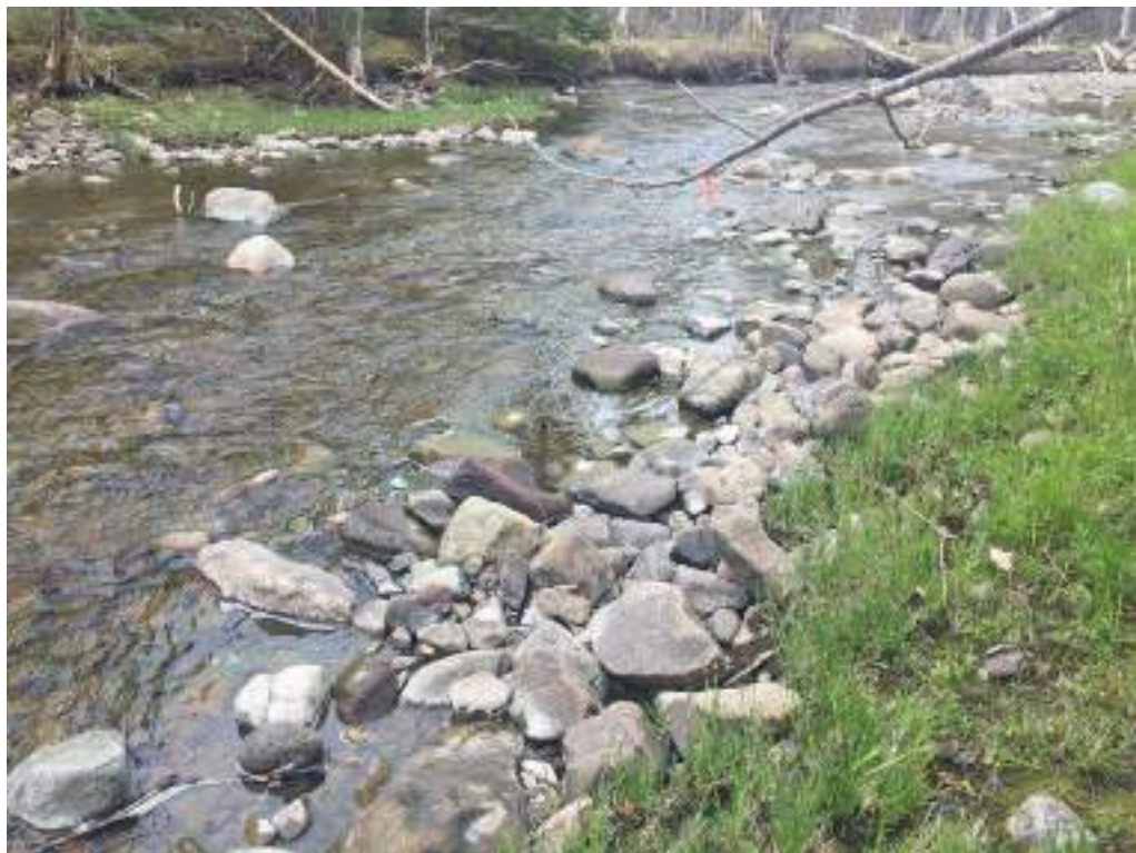
Figure 239. Structure #53 Deflector - requires a full rebuild.
