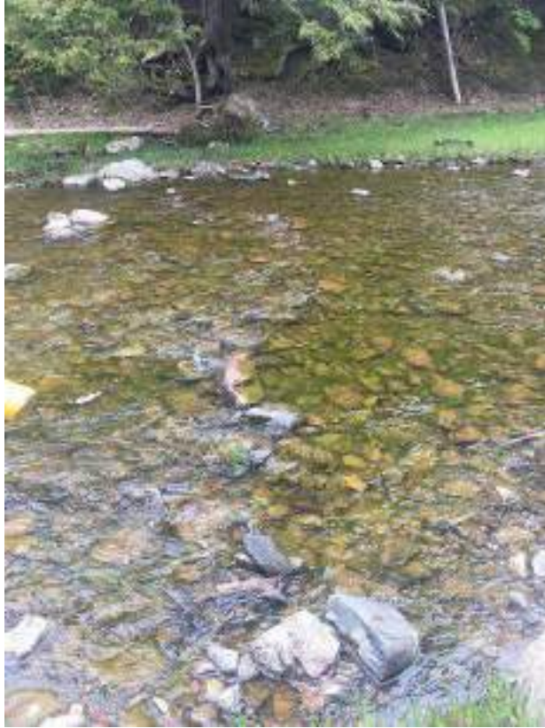
Figure 242. Structure #56 Rock Sill - requires maintenance.
