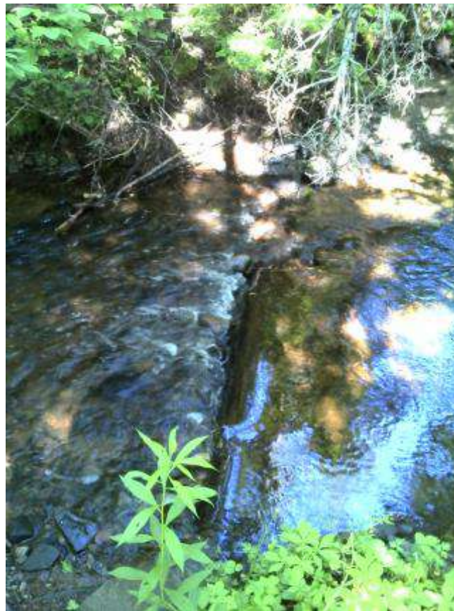
Figure 63. Structure #15 - Before and after picture of the maintenance completed on a digger log.
