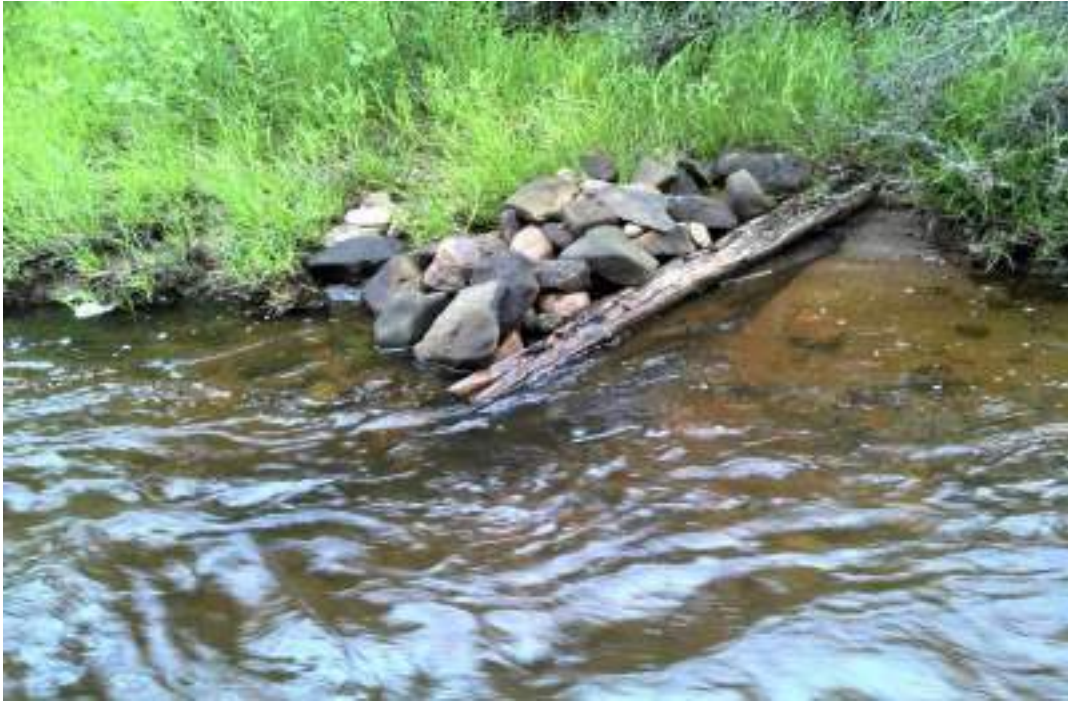
Figure 155. Deflector #8 - after picture of maintenance. The front of the structure is missing and needs to be fixed. Rock was added to help deflect the waterflow from the bank.
