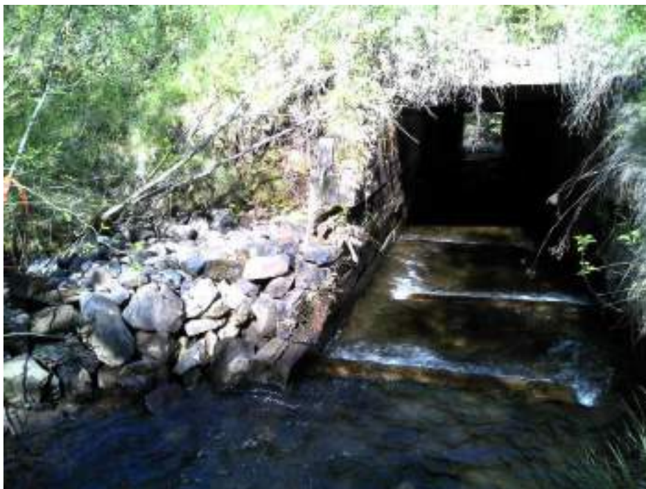
Figure 17. Showing the baffles in the boxed culvert. Rock was added on the left-hand side to avoid any further bank erosion from occurring.
