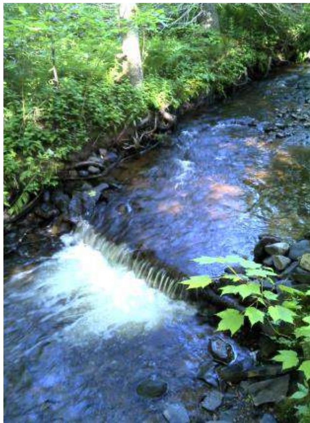
Figure 49. Digger log #1 - furthest structure upstream. Before and after pictures of the completed maintenance.
