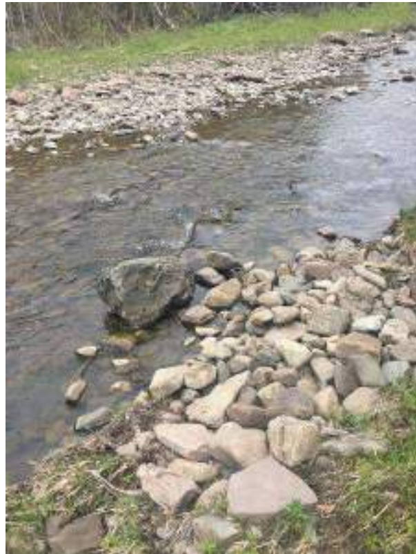
Figure 233. Structure #47 Deflector - requires full rebuild.
