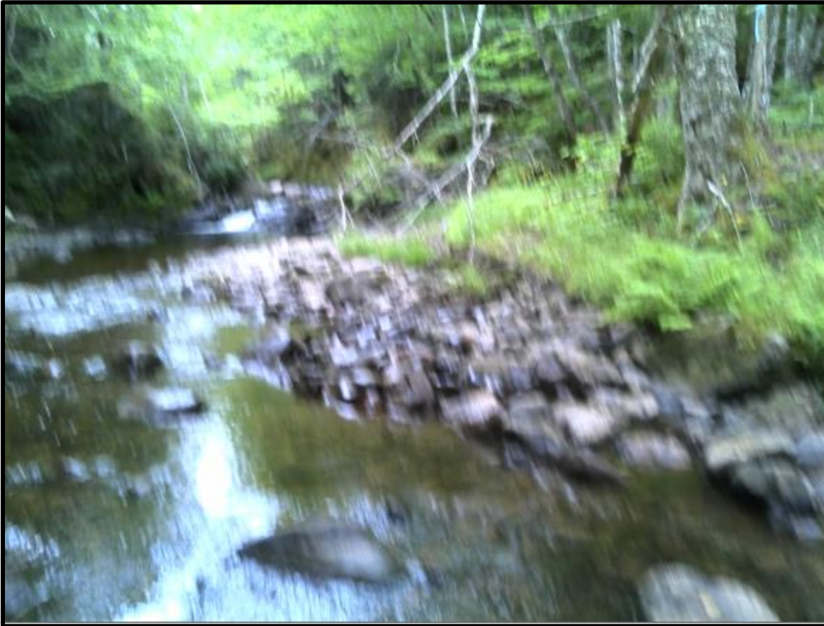
Figure 145. Before picture of deflector at waypoint 190.
