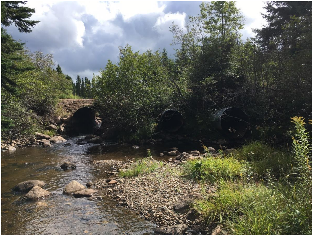
Figure 37: Culvert (Looking upstream) - Remediation required for fish passage
