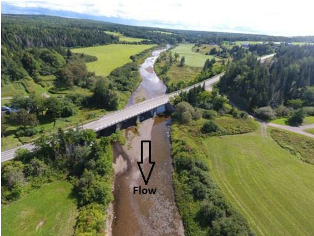
Figure 11: Route 19 Bridge, note scouring below bridge. Over-widened and shallow channel. Potential barrier for early run fall Atlantic salmon. Evidence of ice scouring of spawning habitat and lack of sufficient riparian zone.
