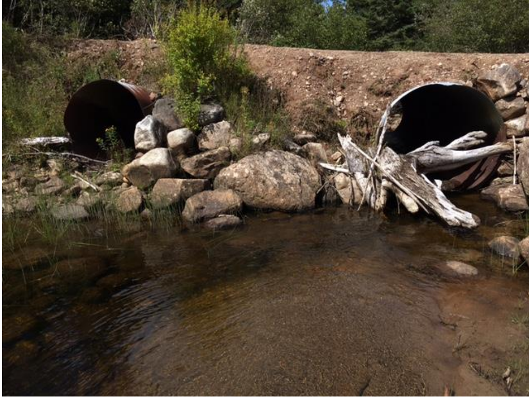
Figure 36: Fish passage barrier - MacLeod Brook (Looking downstream)
