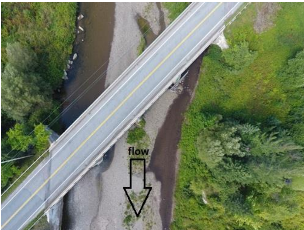
Figure 12: Route 19 Bridge, mid-channel substrate deposits and split channel. Channel is also over-widened.
