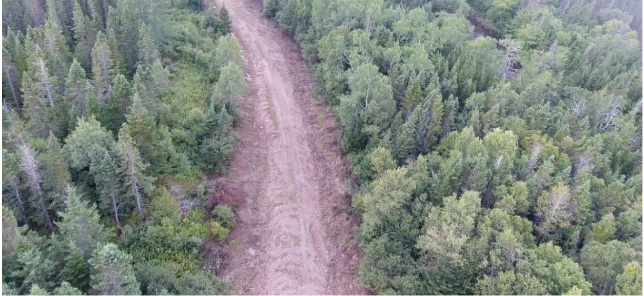
Figure 3: Road and newly constructed ditching leading to fine sediment runoff in MacLeod Brook.
